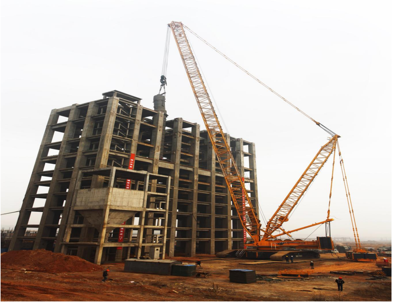
On February 5, 2012, the comprehensive energy coal-to-gas project of henan yima coal industry was under construction
